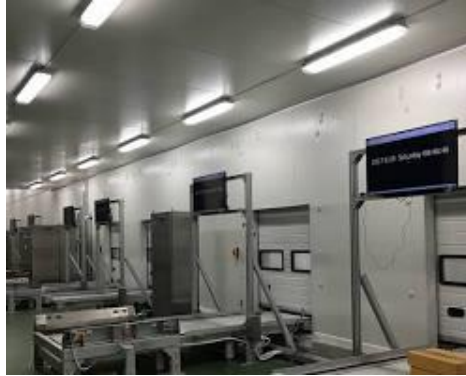
Roller Conveyor in a Cold Storage
