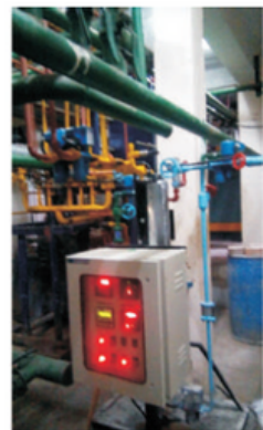
Fully automatic air purger in operation
