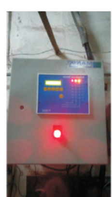
Ammonia Leak detection system
