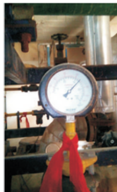
Plant discharge pressure before plant modification
