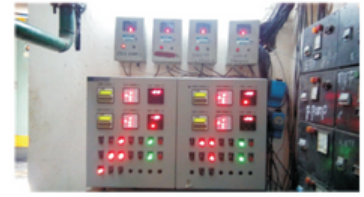
Automatic liquid level control, temperature control and hot gas defrosting system
