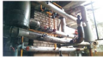
Plant piping before modification
