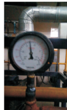
Plant discharge pressure after plant modification
