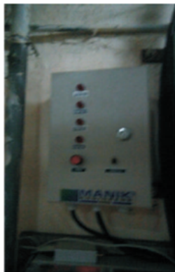
Cold Room Safety
